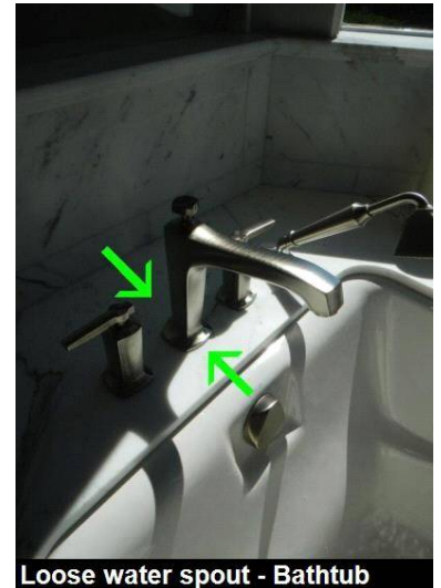
Loose water spout - Bathtub
