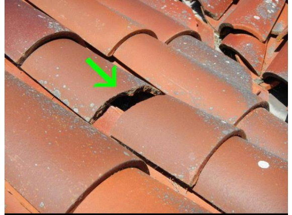
Damaged roof tile
