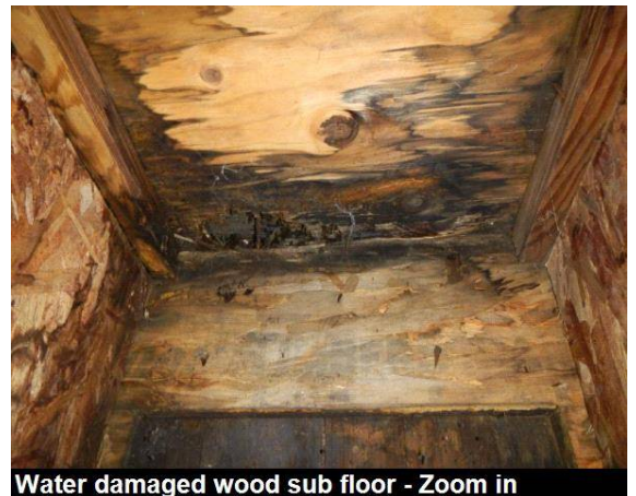
Water damaged wood sub floor - Zoom out
