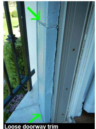
Loose doorway trim
