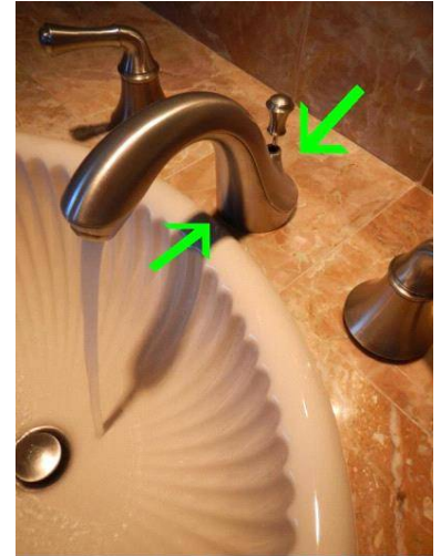
Loose water spout - Sink faucet
