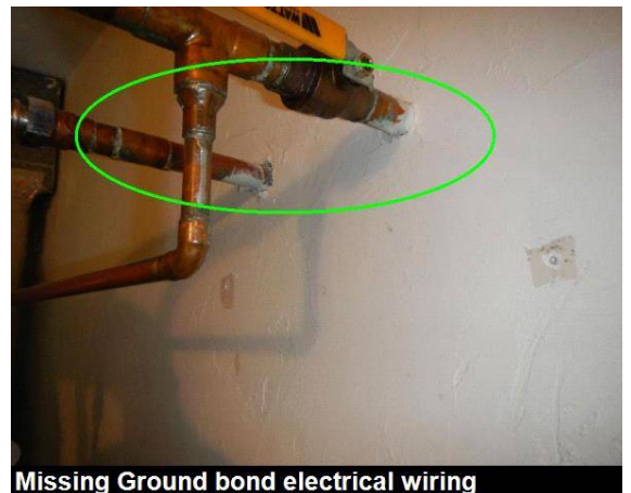
Missing Ground bond electrical wiring
