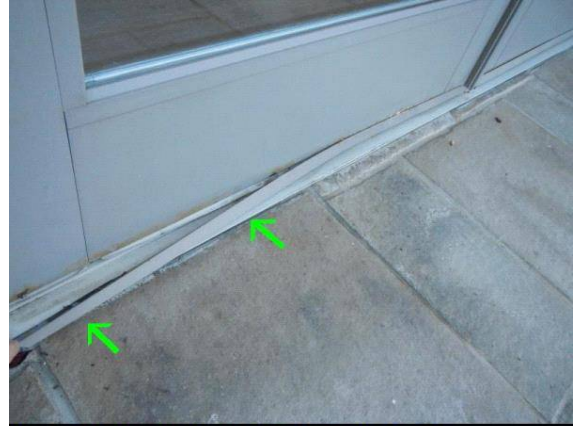
Loose (partially detached) weather seal
