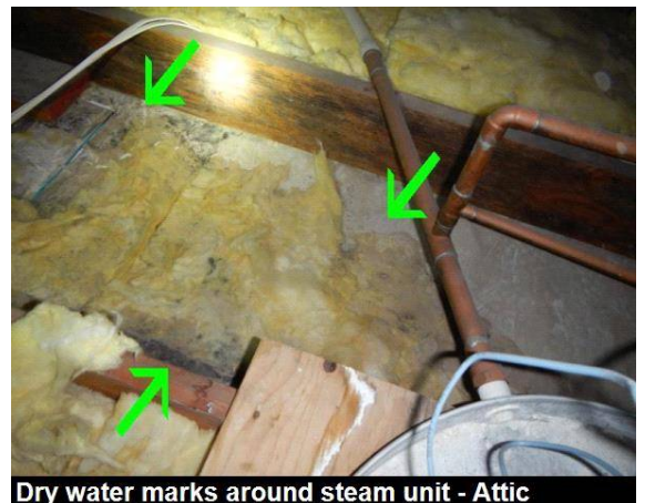
Dry water marks around steam unit - Attic
