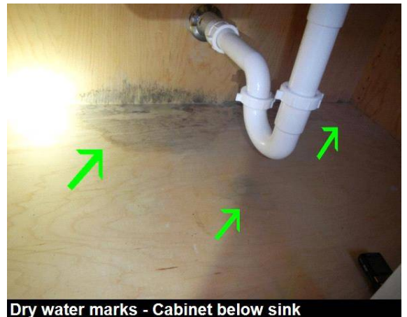
Dry water marks - Cabinet below sink
