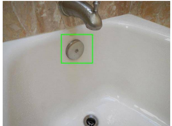
Loose overflow finish plate - bathtub
