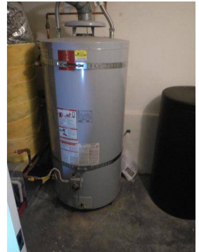
Water heater - Lower level mechanical room
