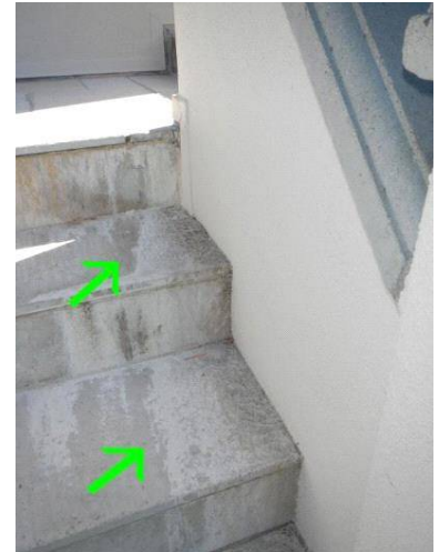
Leached tile sealer - Right side stairway
