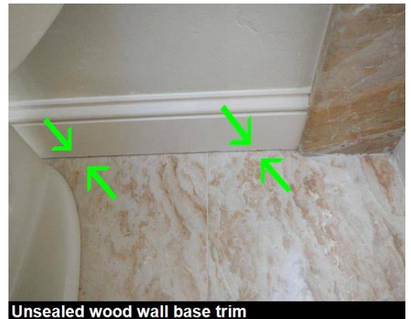
Unsealed wood wall base trim
