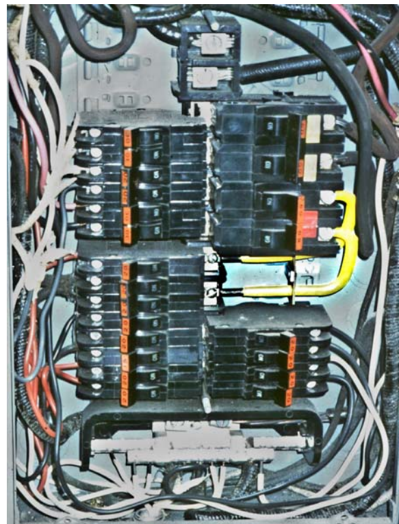
Figure 3 – Split Bus Panel
