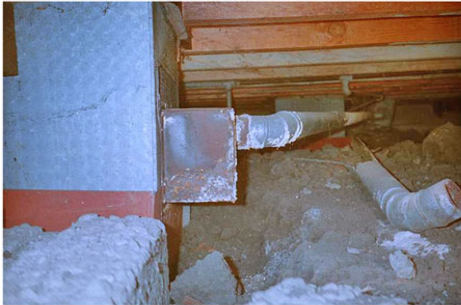
Photo 3 - Rusted Draft Hood and Discarded Old Vent
