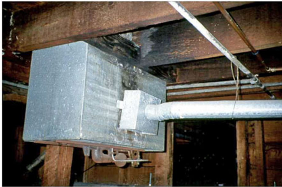
Photo 2 - Loose Draft Hood and Charred Framing
